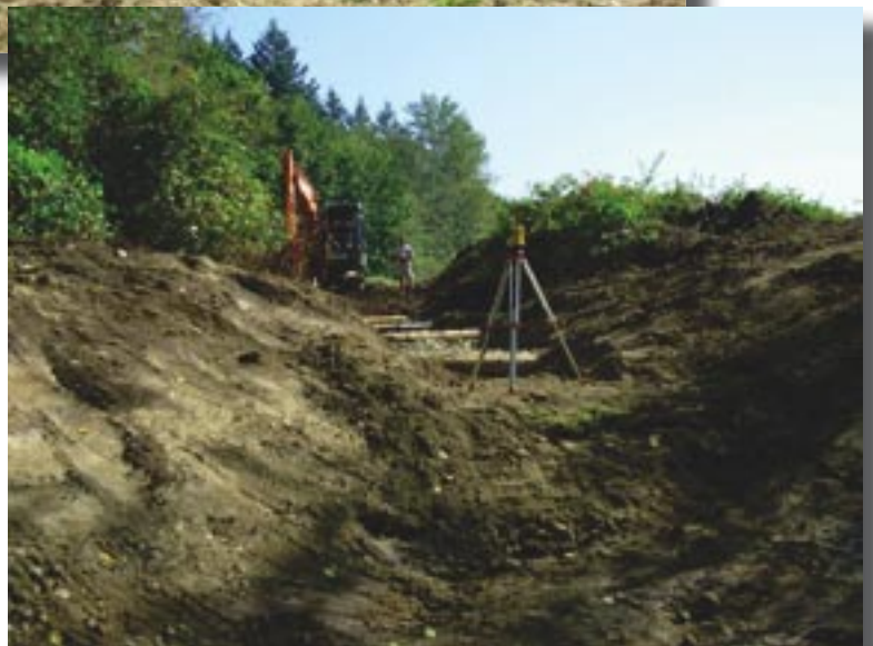
Metamorphosis: First, the old seasonal channel was cleared of blackberry (top), then crews dug out a new profile (above) that would resolve drainage problems and create off-channel habitat for overwintering salmonids (To get a sense of scale, note the person standing next to the backhoe) .
