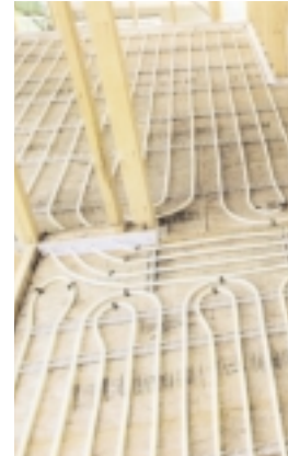
above: EcoCafe radiant floor system
